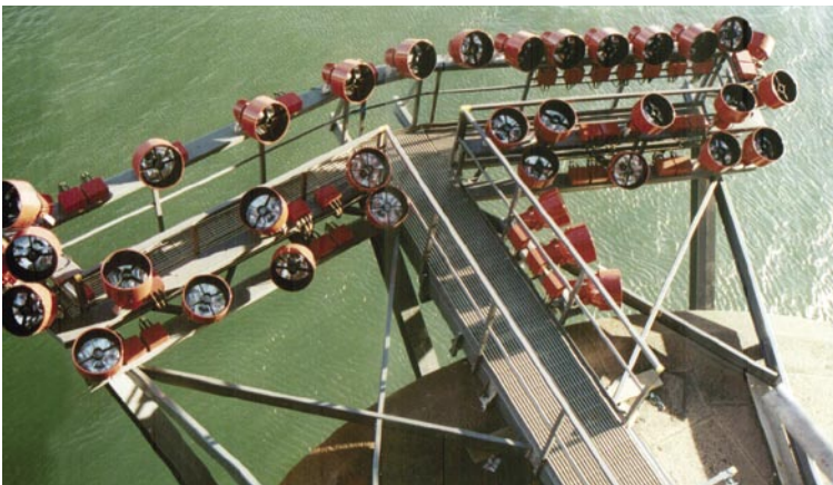
EXTREN® structural shapes were used to fabricate twelve platforms holding the spotlights that illuminate the Forth Bridge in Scotland.
