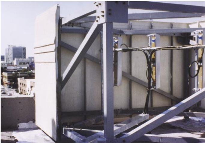
EXTREN® fiberglass plate and structural shapes were used for cellular shielding and were made to match the style and appearance of the Santa Ana Historical building.
