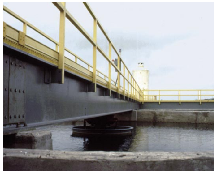
Lightweight, corrosion resistant 24" (610mm) I-beams span 45' (13.7m) to bridge clarifiers at the Las Rusias, Texas Wastewater Treatment Plant.
